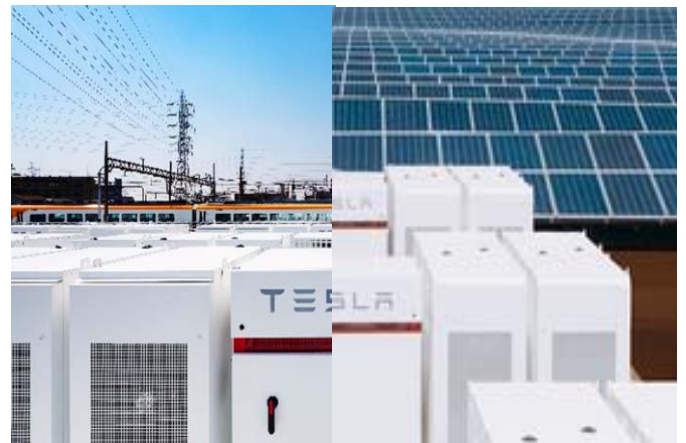
Ex 10: Battery Energy Storage (B-ESS) Applications
