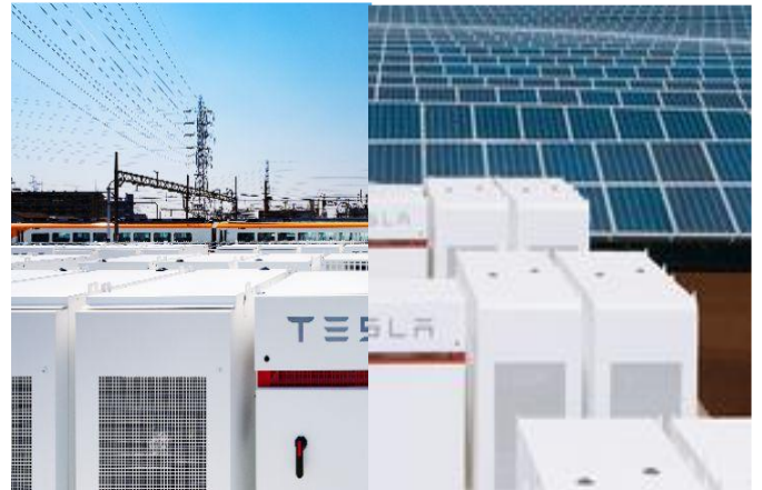
Ex 10: Battery Energy Storage (B-ESS) Applications
